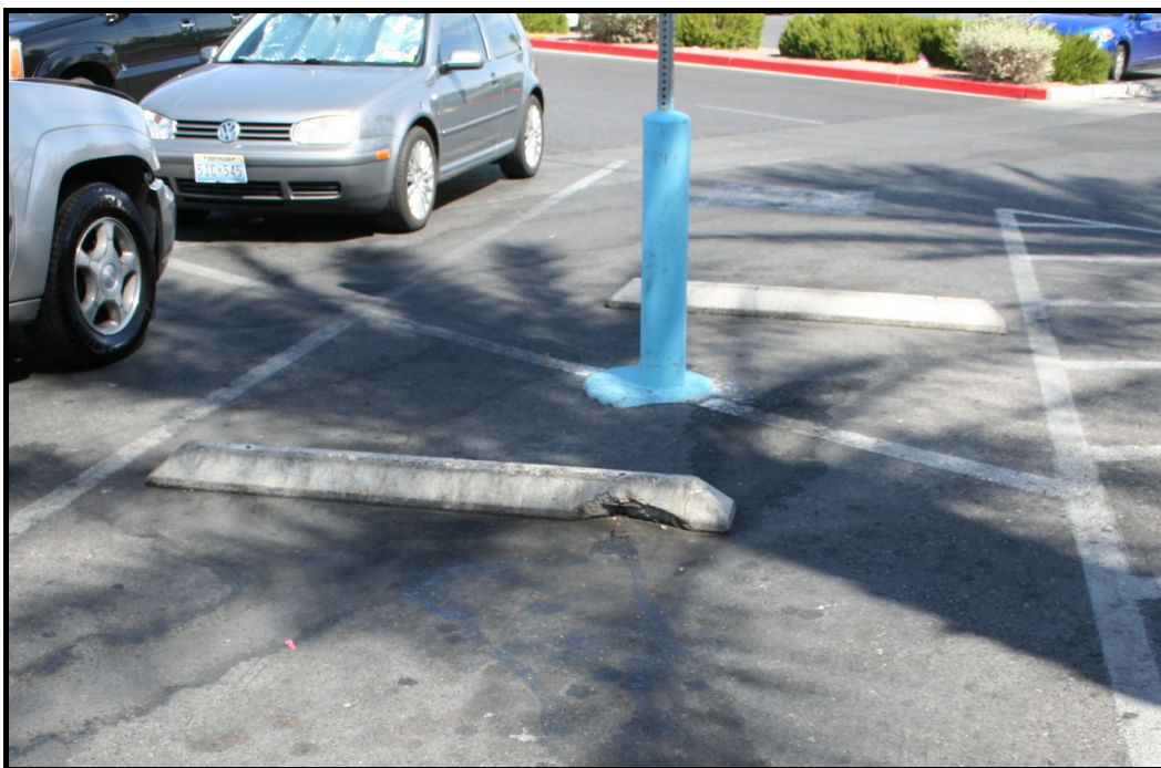
Photo Ex. 1: Note fractured wheelstop.
