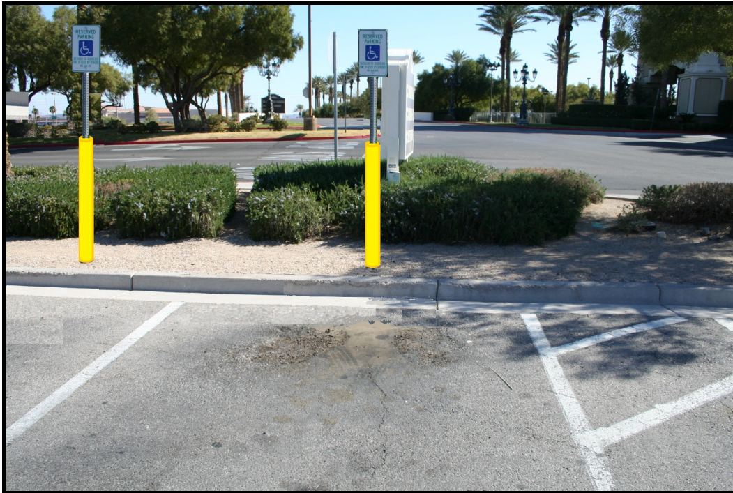
Photo Ex. 5. Wheelstops removed and signs placed atop concrete-filled steel bollards.
