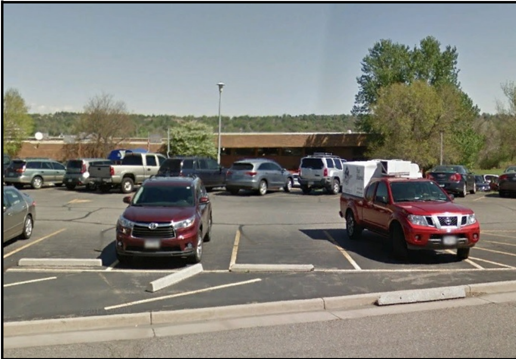
Photo Ex. 2: Note displaced wheelstops.
