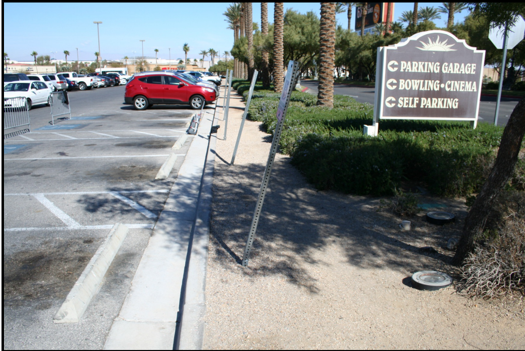
Photo Ex. 3. Note leaning sign posts.
