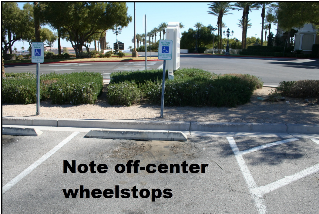
Photo Ex. 4. Off-center wheelstops created tripping hazard.
